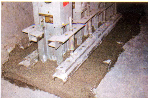
Application for bus duct hole
